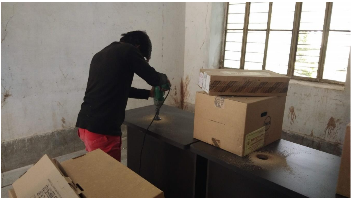
Computer Lab Installation : South Campus,SCRS Rajkiya Mahavidyalaya
